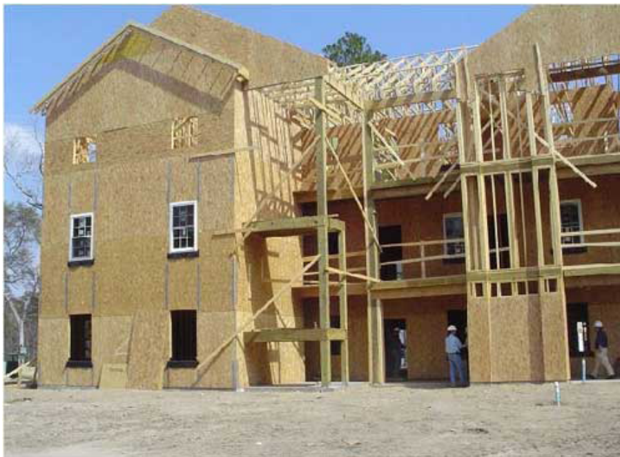
Photo 2 (Case Study 2). This condominium project was the site at which the worker's fatal fall occurred. Photo by SCOSHA.
